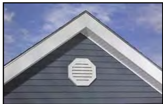
Figure 16 – Example of a faux gable vent for decorative purposes only.
