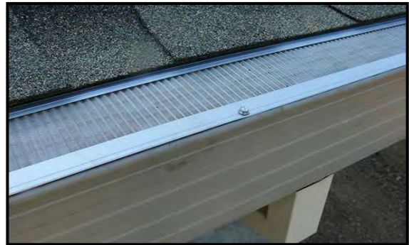
Figure 17 – One example of a gutter cover or guard to protect against debris accumulation.
