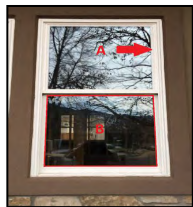
Figure 10 – (A) Double pane window example with proper frame construction and (B) tempered glass pane.
