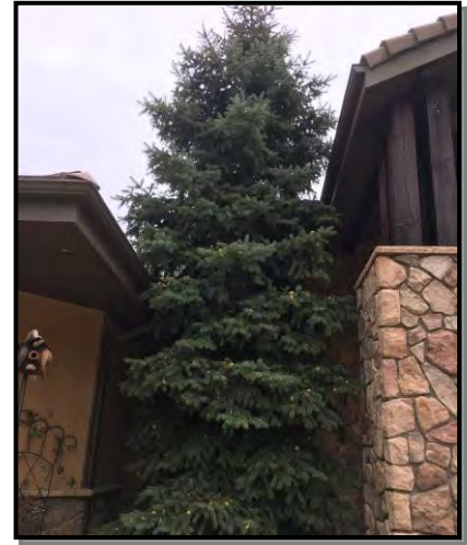
Figure 2 - Example of vegetation that is in close proximity to a structure siding.
