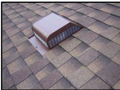
Figure 11 – The 1/8-inch screening can be seen where it contrasts with the wood on the inside of the vent.
