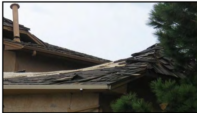
Figure 1 – Example of a shake shingle roof that was ignited from an ember in the 2012 Waldo Canyon Fire.
