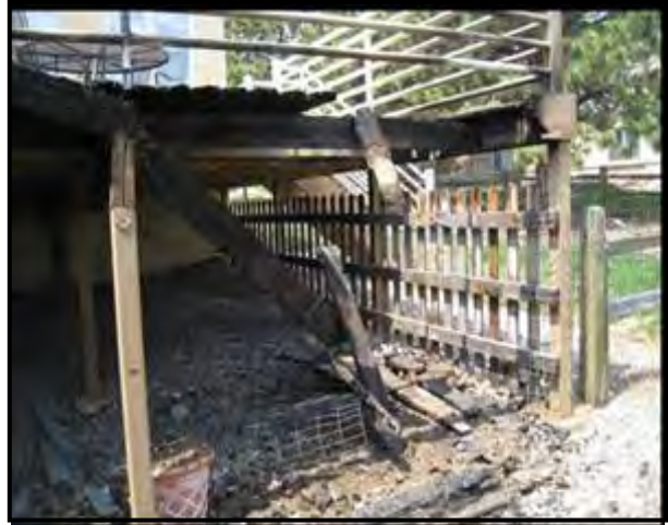
Figure 21 – Example of a wood deck ignition on a wood deck.
