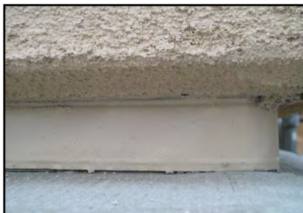
Figure 24 – Example of the base of the siding properly sealed with stucco and flashing to prevent exposure to the base of the house.
